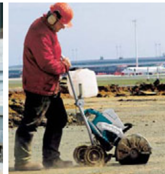
Precision cutting in asphalt with the disc cutter mounted on the saw cart.
